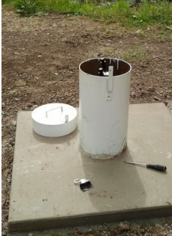
Above ground housing w/ lockable cap
